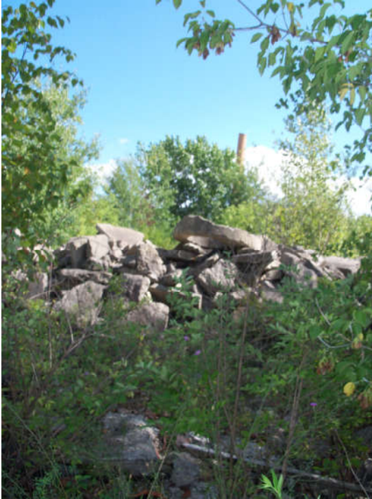
Photograph 6: Rail Yard Debris; A concrete floor and piles of broken concrete several inches thick remain at the site of the former Roundhouse, as well as some of the foundation. The smoke stack, approximately 160 feet tall, is visible at the rear of the photo.
