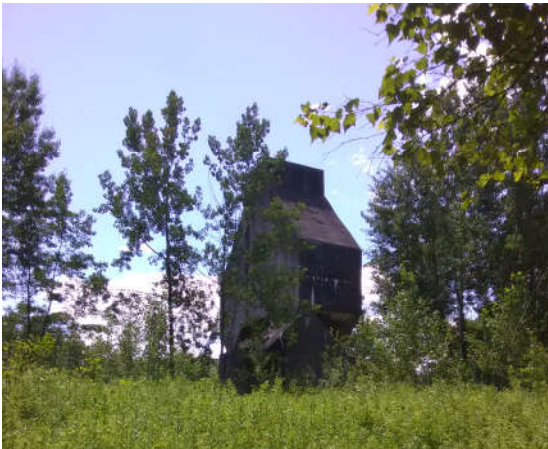
Photograph 7: Rail Yard Concrete Structure; An 80-ft structure formerly utilized to load coal and sand into rail cars (coaling tower).
